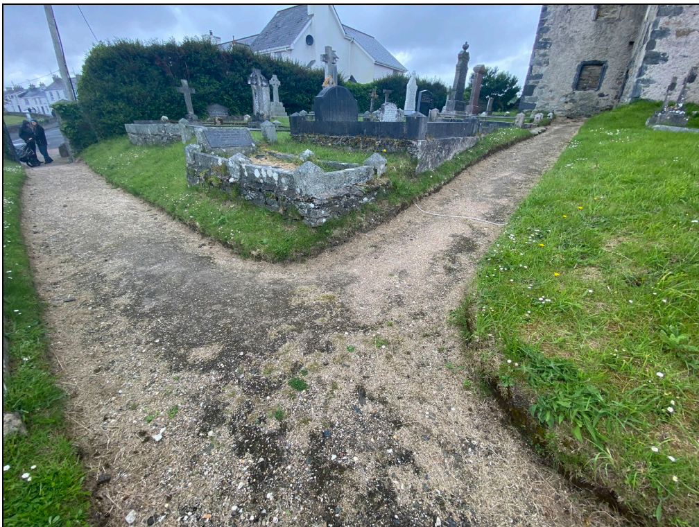
Plate 17: NW facing view of the existing footpaths within the graveyard which are proposed to be upgraded.
